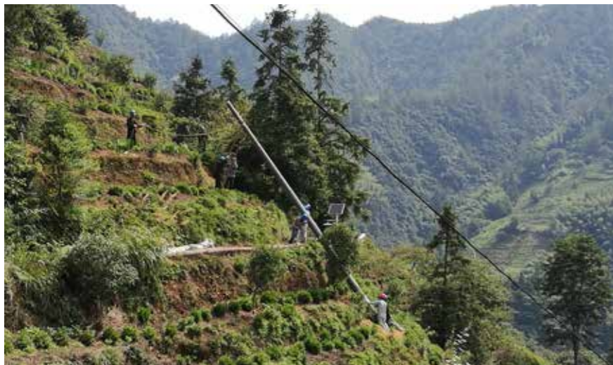
Composite utility poles significantly shorten the time of power supply repair in Huangshan, Anhui province. In the photo, several workers are transporting the new composite pole.
